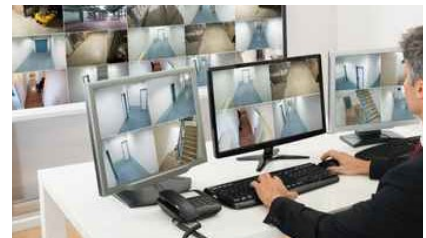
Central management platform
